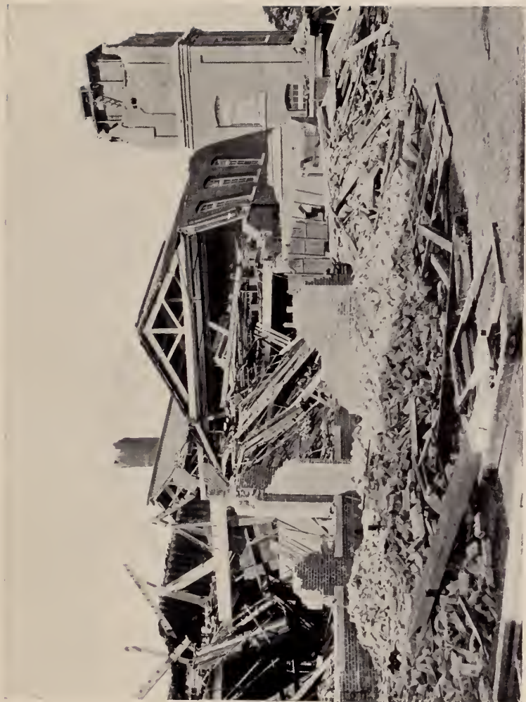
WRECK OF COTTON FACTORY, NAGOYA, JAPAN, BY THE EARTHQUAKE OF 1891
